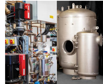
HVAC Data Centre cooling
