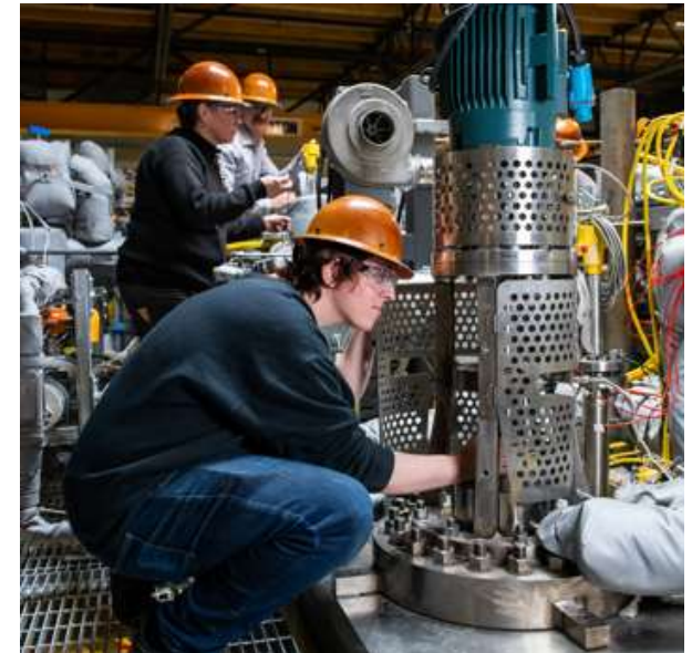
TerraPower technician with HT molten salt pump
